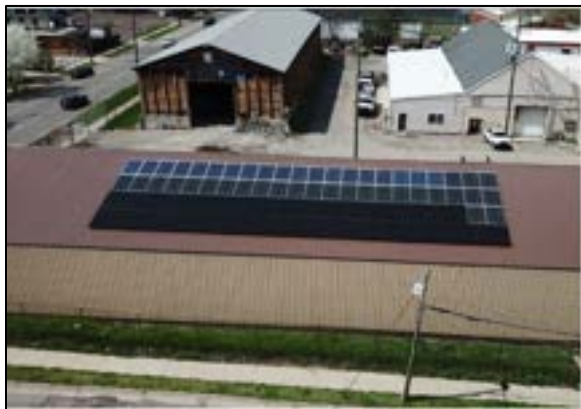
Figure 1. Solar array Installation on City of Ypsilanti Department of Public Service carport. Source: solarypsi.org
