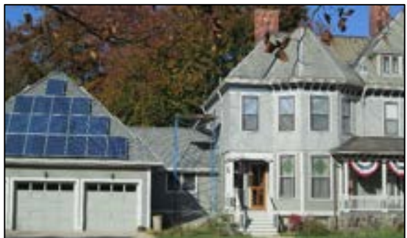
Figure 3. Solar array installed on historic property in City of Ypsilanti. Source: City of Ypsilanti.
